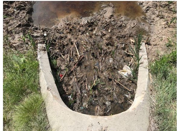
Sediment was not removed from inlet pipe – South Pond, north inlet.
