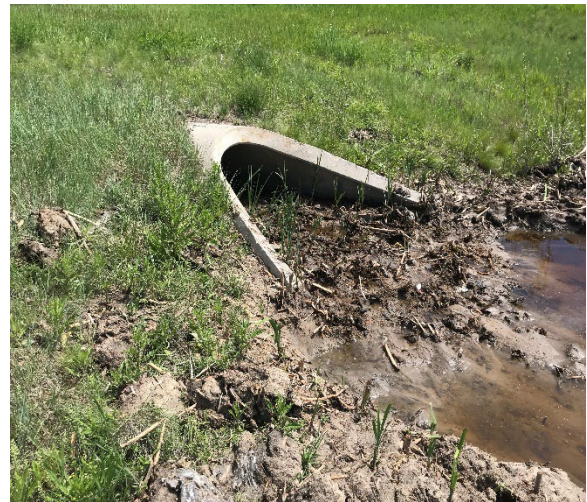
Sediment was not removed from inlet pipe – see photo above also.
