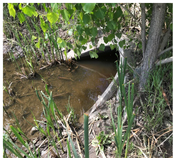
Sediment was not removed from inlet pipe – North Pond, west inlet.
