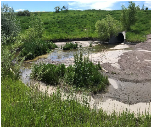
Sediment and vegetation was not removed from inlet forebay – North Pond, south inlet.
