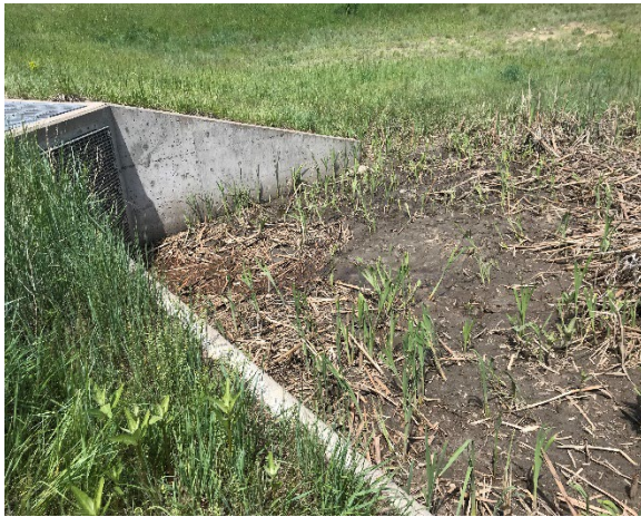
Cattails appear to have been cut but sediment was not removed from concrete pad in front of outlet – South Pond outlet.
