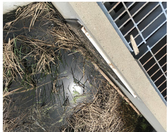
Trash rack needs scraped off – North Pond outlet.
