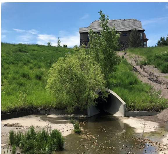
Tree adjacent to inlet needs to be removed – North Pond, south inlet.
