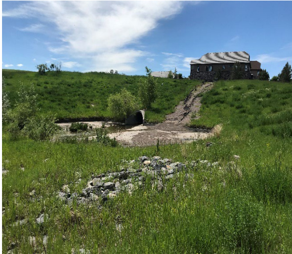
Maintenance access road was not repaired. North Pond, south side.
