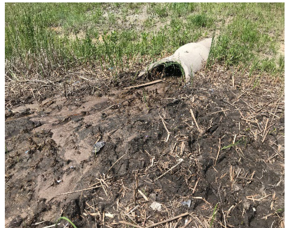
Sediment was not removed from inlet pipe – South Pond, west inlet.
