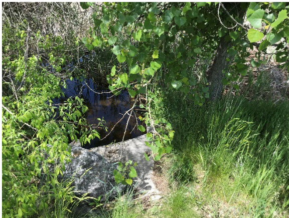
A tree adjacent to concrete inlet pipe is needed – South Pond, east inlet.
