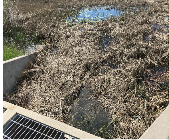
Cattails and sediment removal from concrete pad in front of outlet was not done – North Pond outlet.
