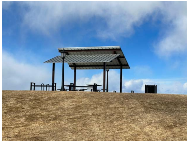
This is for the replacement of the metal shade structure located at the Hilltop Park.
